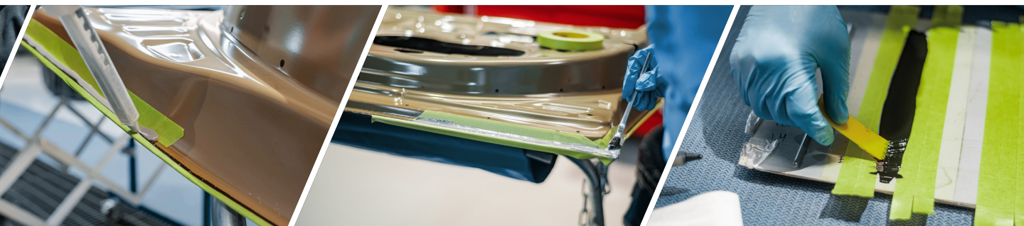
Toyota Collision Repair Technical Trainer displays the proper techniques when applying adhesives. Always refer to TIS techninfo.toyota.com for specific recommended procedures.
